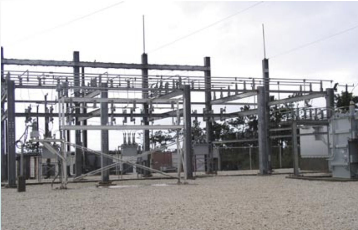
The Substation connecting Independence Village to the National Grid was completed in July 2003 under the Power IV Project.
