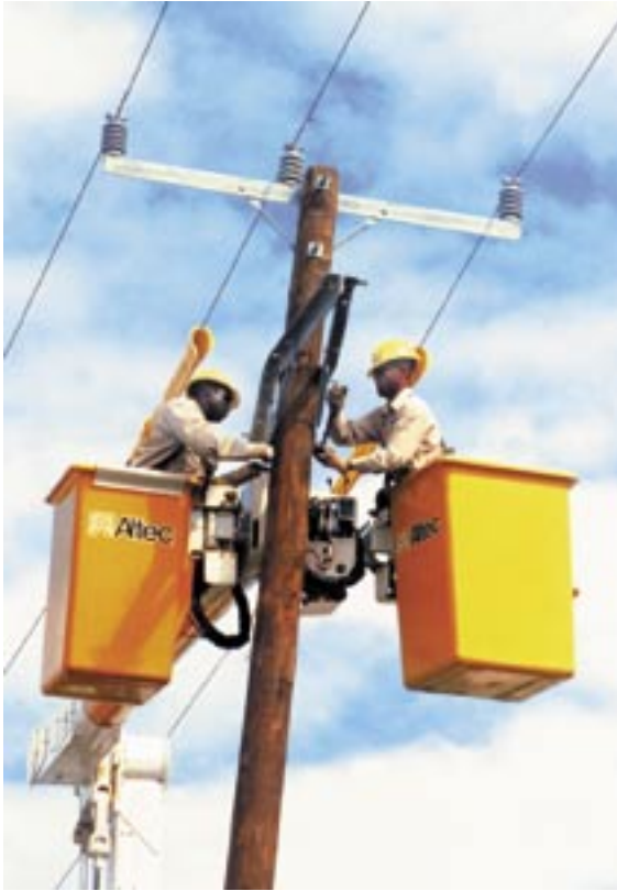
Linemen outfitting a new pole structure as part of the Reliability Improvement Project (Power V), which was initiated in 2003.
