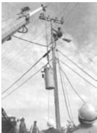
Heavy load: BELCO workers use a crane to lift a replacement transformer into position on this pole along Marsh Folly Road ■ Photos by Patrick Bean
