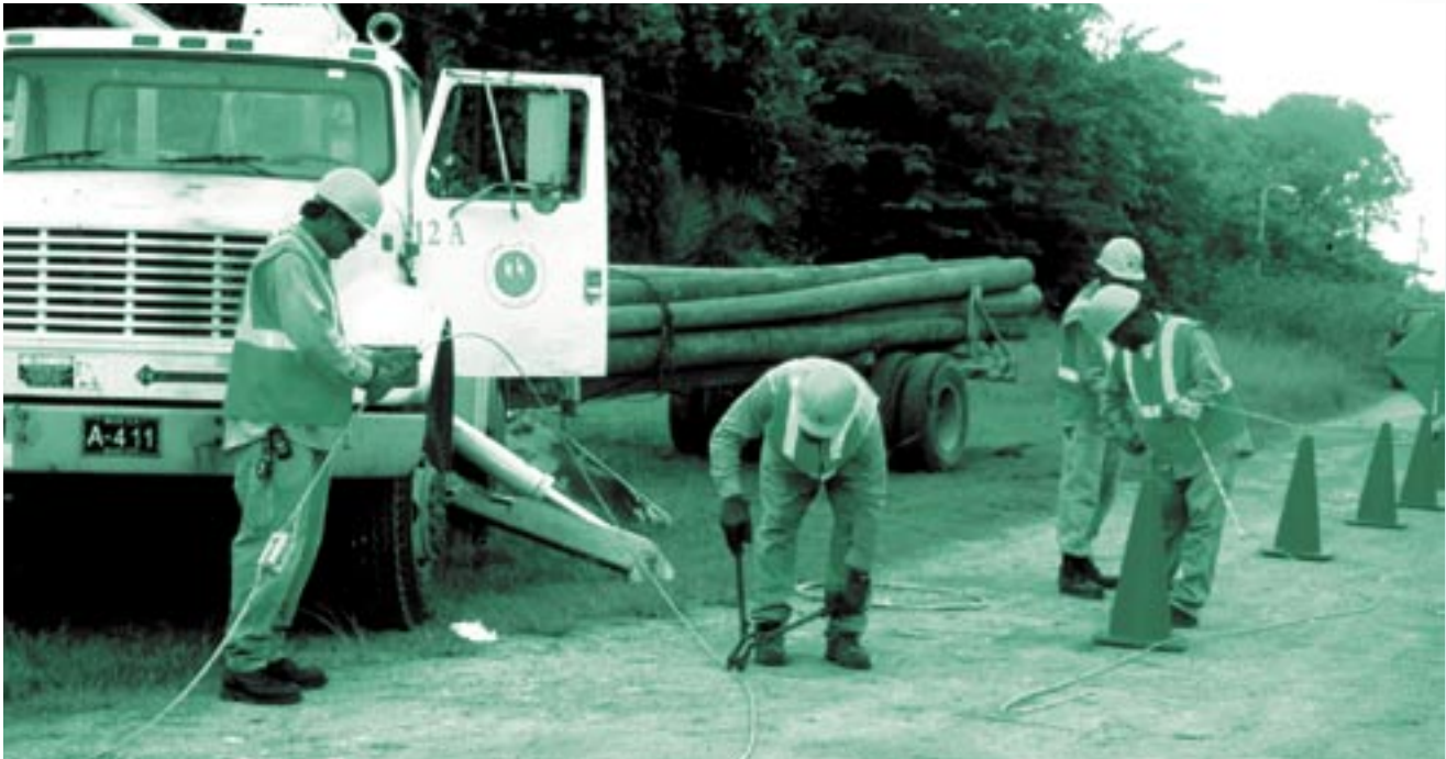
A BEL line crew constructing power lines under the rural electrification component of the Power III Project. This project contributed to increased sales growth.
