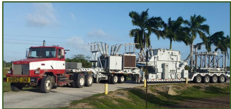
BEL's mobile substation
