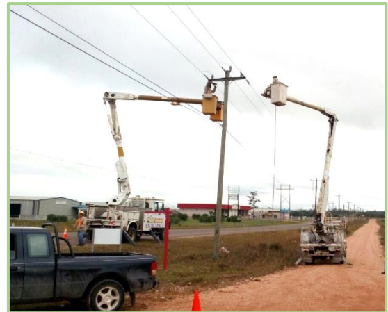
New power lines being energized on Iguana Creek Road to supply Selena, Santa Teresita, Los Tambos and San Marcos Villages.
