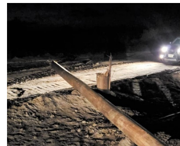
Pole broken by excavator
